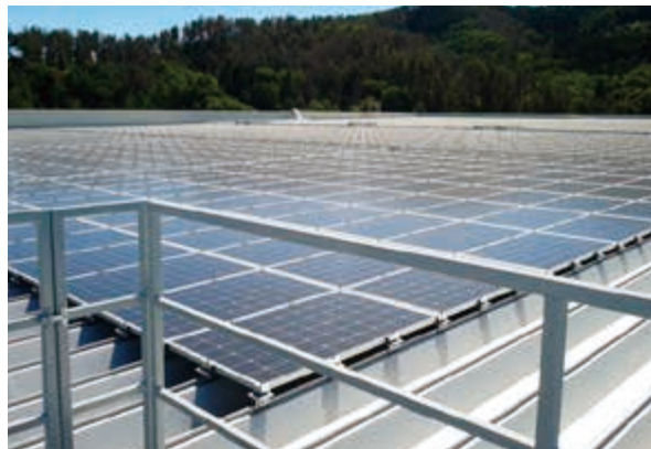
Solar panels at Fujiyama Works
