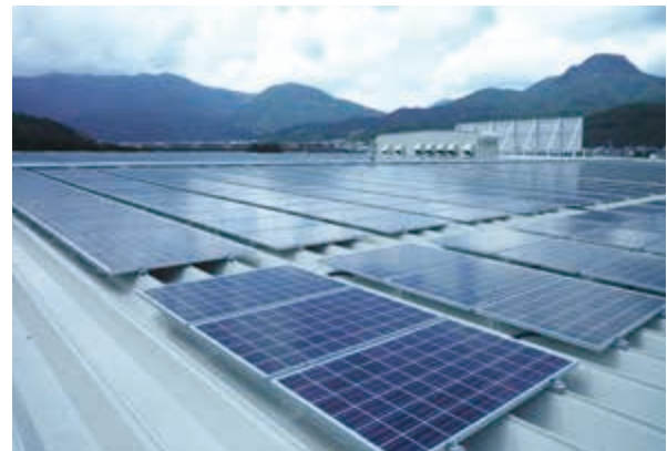
Solar panels at Logistics Center
