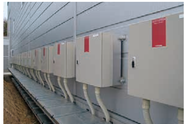
PV Inverters at Fujiyama Works
