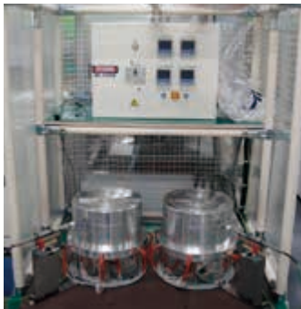
Typical electrical heating system
