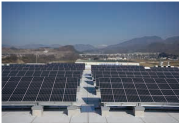
Solar panels at Kangawa Works
